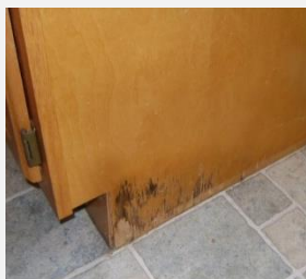
OLD DAMAGE W/MOLD
