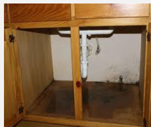
UNDER CABINET LEAKS
